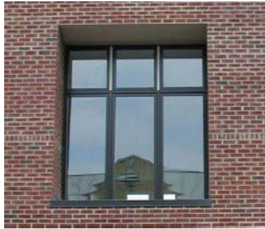
No lintel, arch, or soldier course above a window opening
