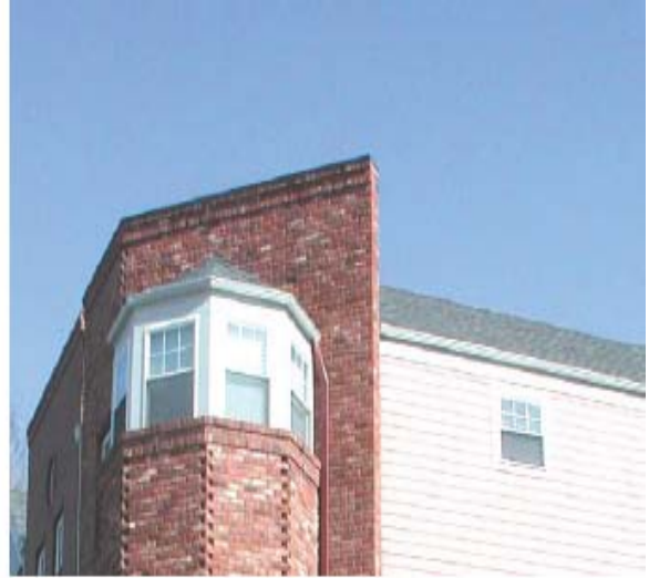
The cornice on this building front does not wrap around the corner at least 4'.
