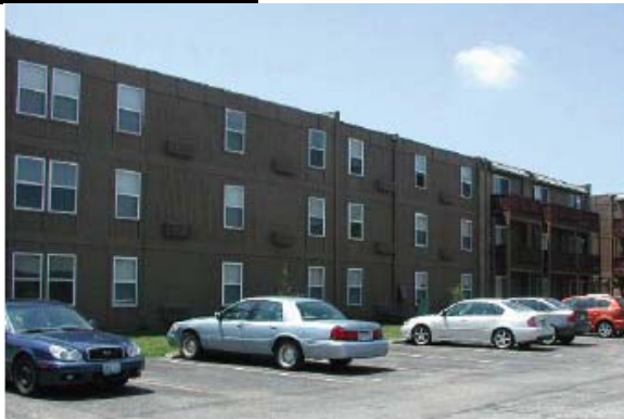
This long wall does not contain offsets at least every 50 feet.
