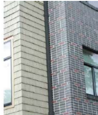
This vertical change in material is done correctly; it occurs at an interior corner
