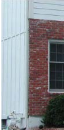
A vertical change in material occurs within 4 feet of an exterior corner.
