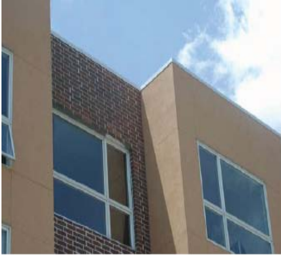
Flashing on top of the parapet does not count as a cornice on building fronts.
