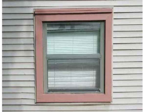
This double hung window is not vertically proportioned.
